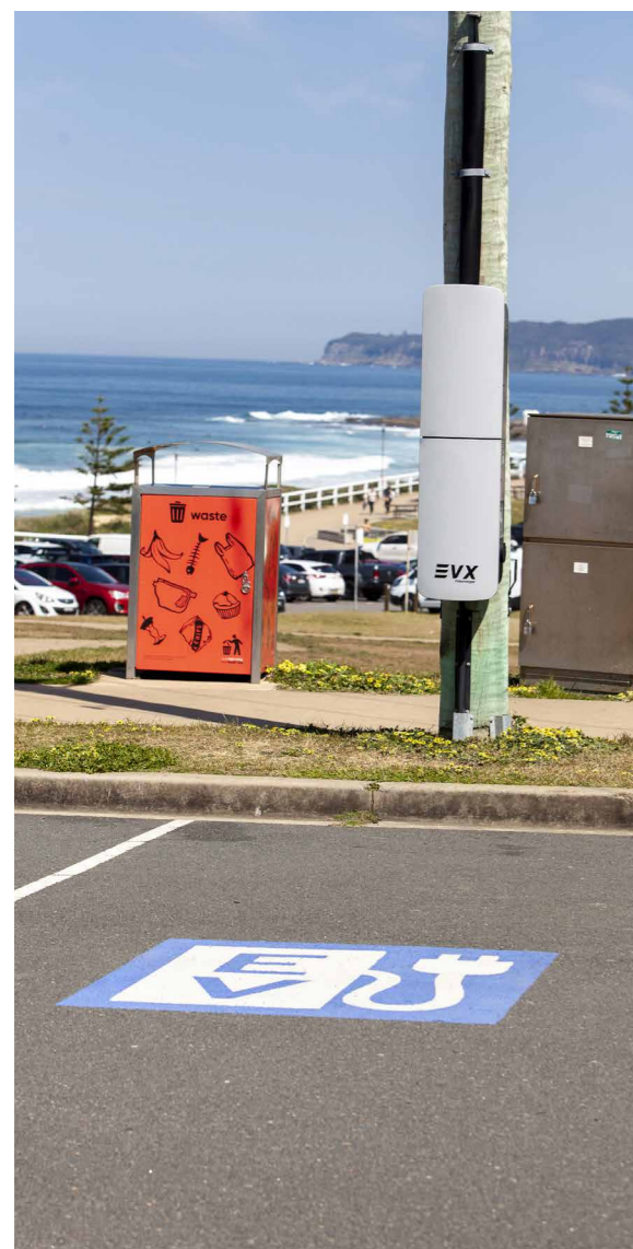
Pole-mounted EV charger at Dixon Park Beach
