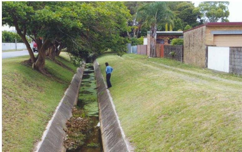
Photo 6: Shows concrete lined stormwater channel at Darling St, in the Cottage Creek catchment. Green organic matter/algae and weed growth is noted in this section of the channel. Sediment accumulation is also an issue within this and other catchments, and other concrete lined stormwater channels.
