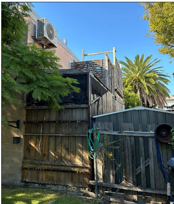
Figure 4 - View of unauthorised decking and boundary works proposed to be demolished (taken from rear yard of 52 Bourke Street Carrington).
