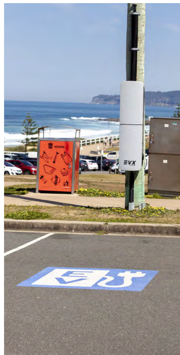
Pole-mounted EV charger at Dixon Park Beach
