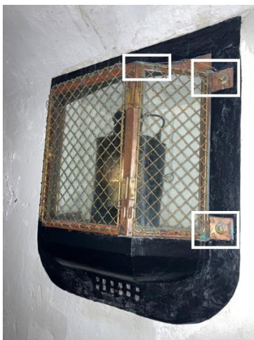
Figure 213. Restored bronze lamp recess displaying minor oxidation. (Source: CPH, 2023)
