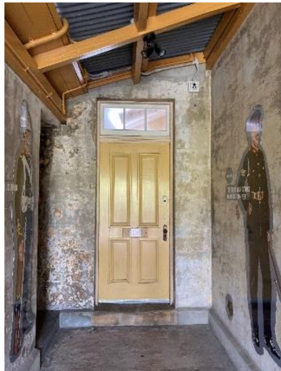
Figure 137. View of four panel door with transom lights leading to pantry room. (Source: CPH, 2023)
