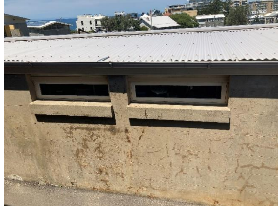
Figure 143. The NCOs' Ablutions are lit by a pair of clerestory windows on its northern elevation. (Source: CPH, 2023)
