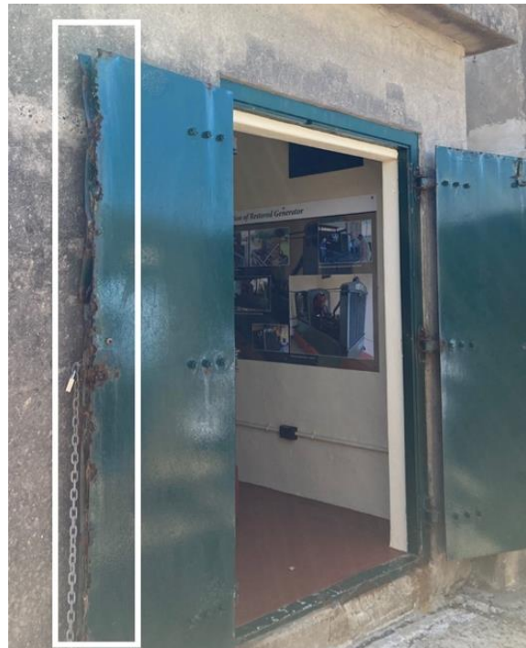
Figure 210. The external doors to the Searchlight Generator Room exhibit signs of deterioration with peeling paint, rust and delamination of the metal sheets from the door leaf. (Source: CPH, 2023)
