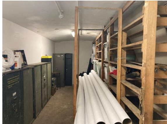
Figure 174. Internal view of western batching room. (Source: CPH, 2023)
