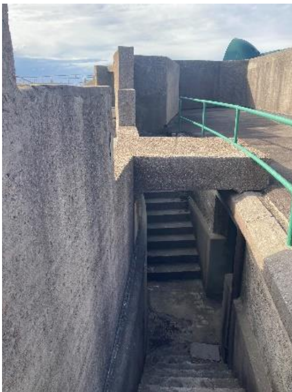
Figure 189. A flight of stairs offers circulation between the gun pits and the blast wall. (Source: CPH, 2023)
