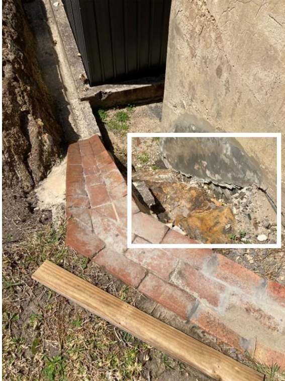
Figure 203. Detailed view of delaminated render and exposed masonry. (Source: CPH, 2023)
