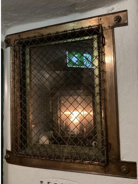
Figure 163. Example of a lamp enclosure contained within the tunnel wall. (Source: CPH, 2023)
