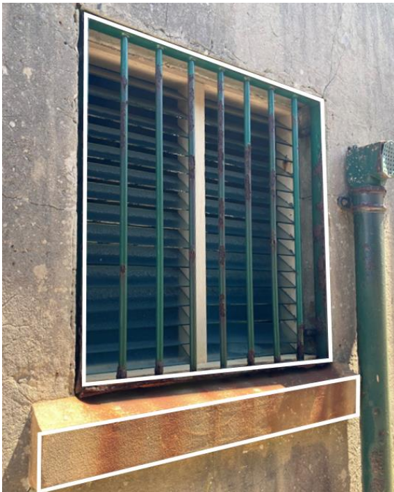
Figure 209. Rusted security bars with peeling paint, causing staining to the projecting sill. There are also signs of lichen growth around the windows. (Source: CPH, 2023)
