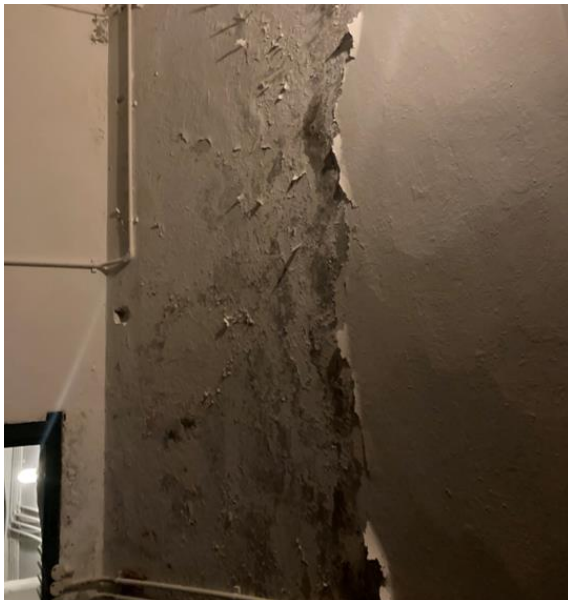
Figure 218. Peeling paint on ceiling of eastern casemate magazine. (Source: CPH, 2023)
