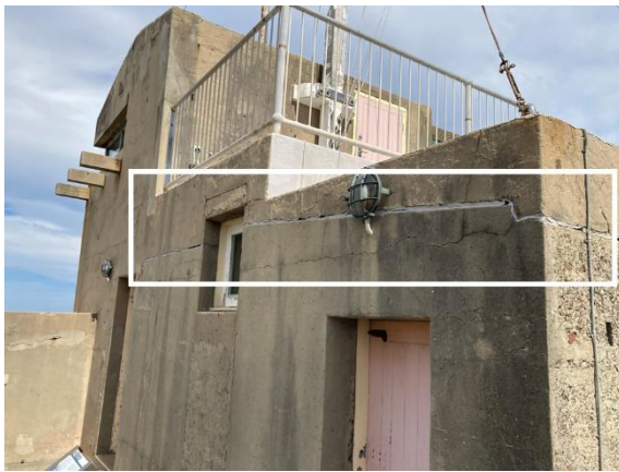
Figure 197. Detailed view of cracking and previous repairs on Battery Observation Post. (Source: CPH, 2023)
