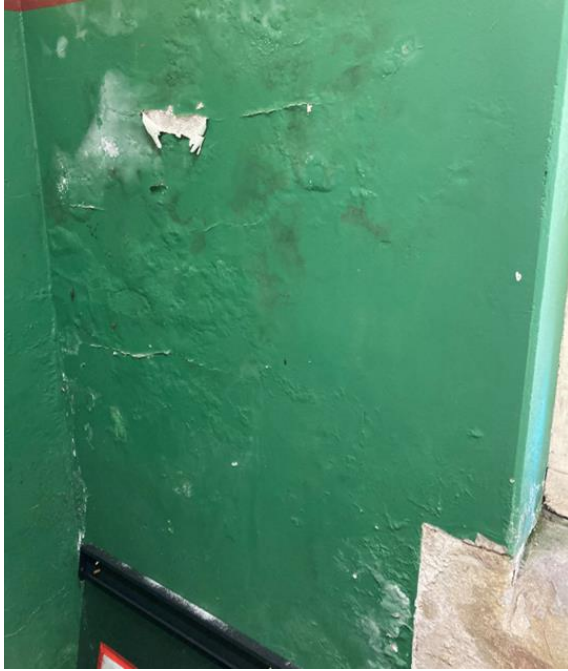
Figure 216. Blistering paintwork with some paint peeling. Salt accumulation is also visible. (Source: CPH, 2023)
