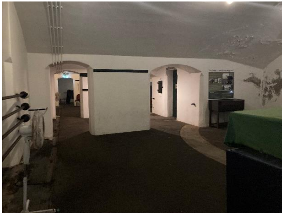
Figure 165. Internal view of the northern casemate battery chamber, looking west. (Source: CPH, 2023)
