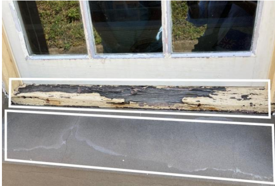
Figure 207. Detailed view of water staining and wood rot present on window sills. (Source: CPH, 2023)
