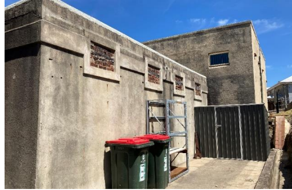
Figure 92. View of rear of Laboratory building. The ventilation units were in-filled with bricks at an unknown time. (Source: CPH, 2023)
