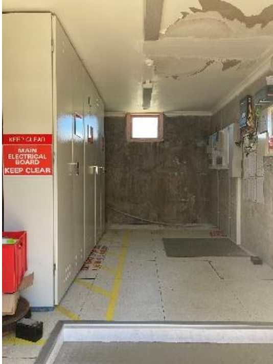
Figure 108. Switchboard and meters in the central stores space. The floors are tiled. (Source: CPH, 2023)
