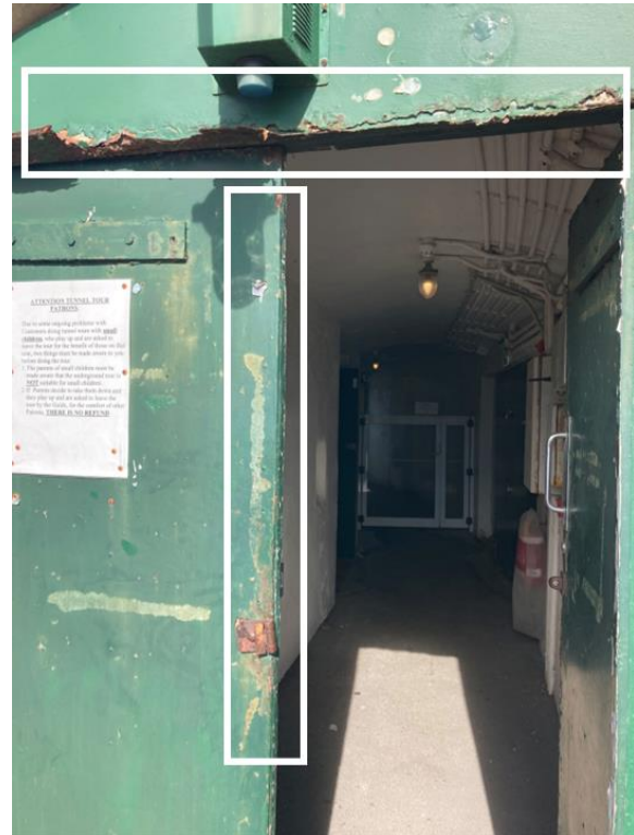
Figure 212. Deterioration of door lintel with peeling paint and rusted metal elements. The door leaves also exhibit peeling paint and rusting. (Source: CPH, 2023)
