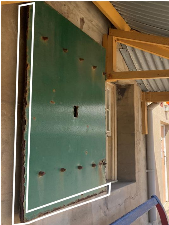
Figure 211. Paint delaminating from the rusted steel shutter. (Source: CPH, 2023)
