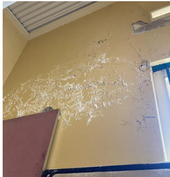
Figure 219. Visible salt accumulation and flaking paint on interior wall. (Source: CPH, 2023)
