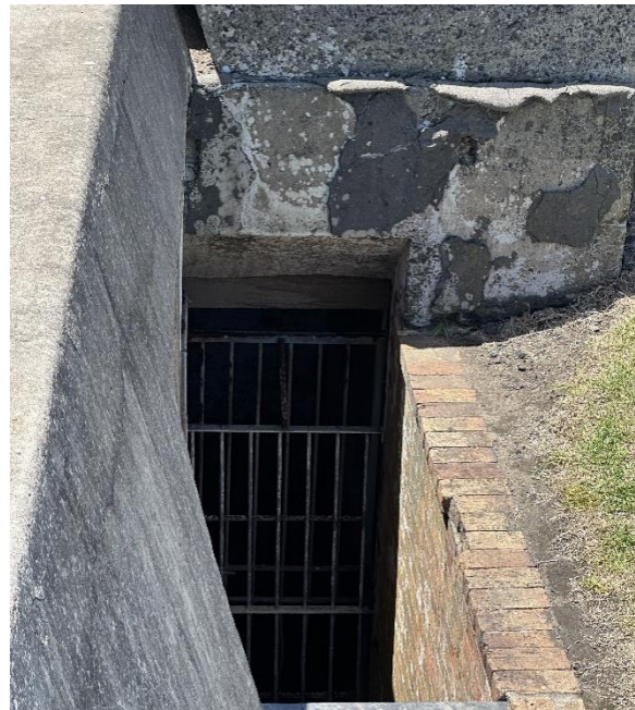
Figure 80. View down Mine Firing Station stairs. The entrance door is currently welded shut due to vandalism concerns. (Source: CPH, 2024)
