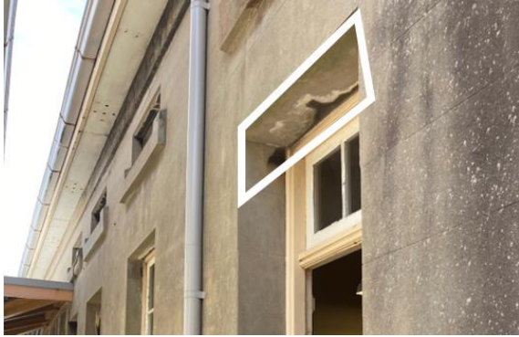
Figure 199. Detailed view of efflorescence and biological staining on NCOs Quarters southern elevation. (Source: CPH, 2023)
