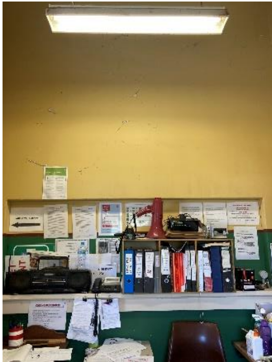
Figure 118. Serving hatch located in Gunners' room. It was filled in at an unknown date. (Source: CPH, 2023)
