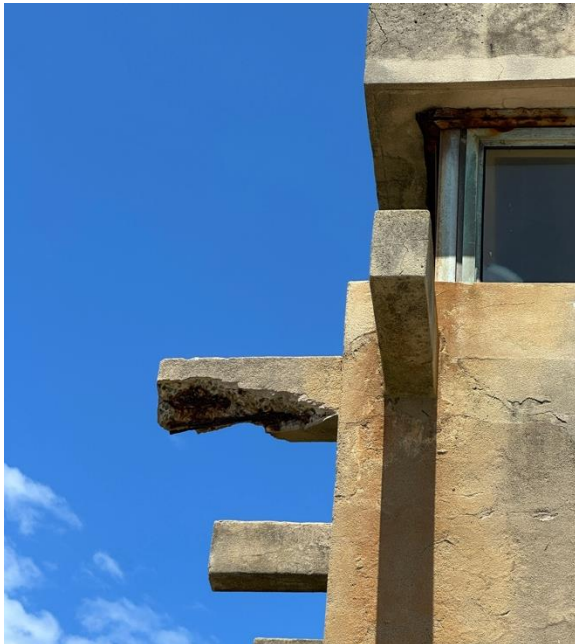
Figure 205. Spalling is evident on Battery Observation Post concrete outrigger. Note the exposed rusted reinforcements. (Source: CPH, 2024)
