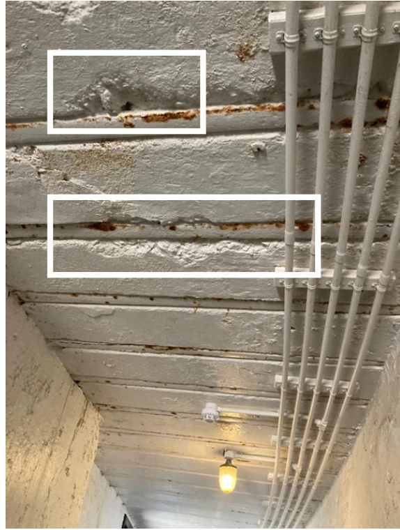
Figure 202. Detailed view of spalling of tunnel ceiling. Note the surrounding rusted elements. (Source: CPH, 2023)
