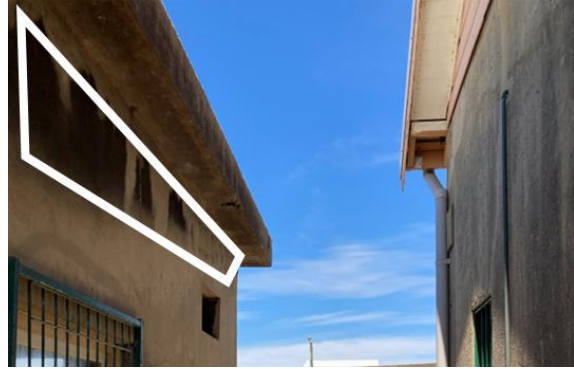
Figure 200. View of biological staining on Searchlight Generator Room western elevation. (Source: CPH, 2023)
