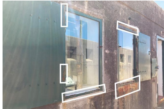
Figure 208. The Laboratory building's windows exhibit rusting of metal elements and deterioration of the window frames. Subsequent rust staining of the façade is evident. (Source: CPH, 2023)
