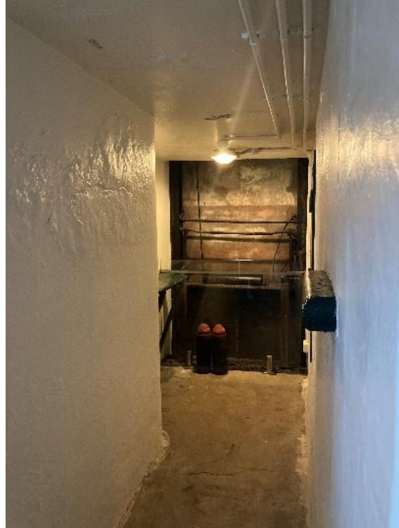
Figure 160. View to lift machine space. (Source: CPH, 2023)
