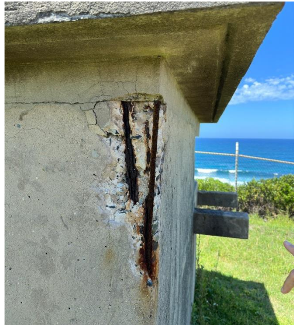
Figure 206. Evidence of spalling at the Searchlight Directing Station. As with the Battery Observation Post, the embedded reinforcements are exposed and heavily rusted. (Source: CPH, 2024)
