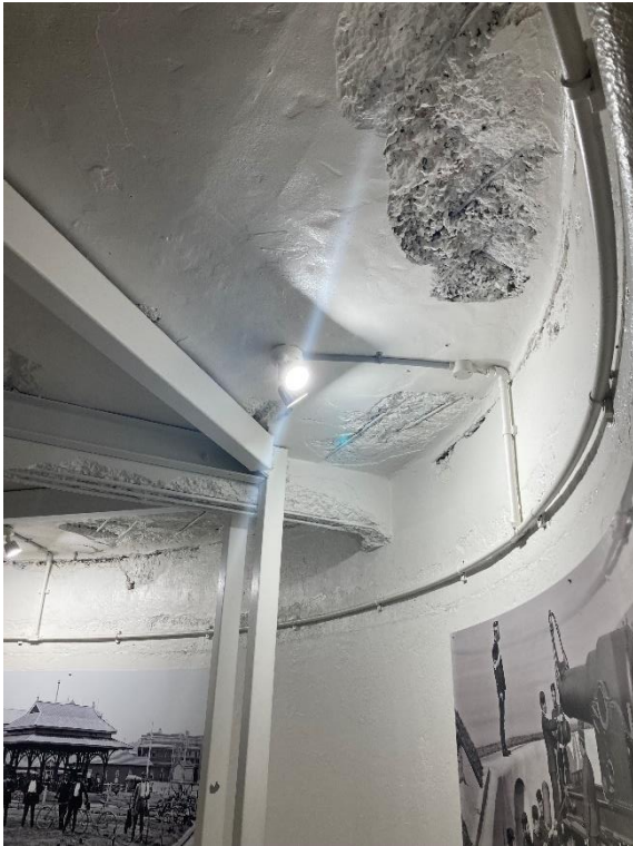
Figure 201. Detailed view of spalling of the ceiling. (Source: CPH, 2023)
