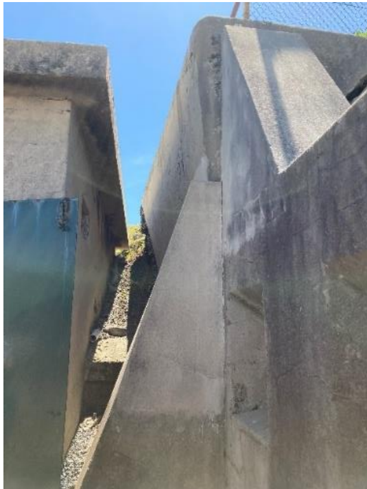
Figure 101. View of the Searchlight Generator Room and dry ditch wall, looking southeast. (Source: CPH, 2023)
