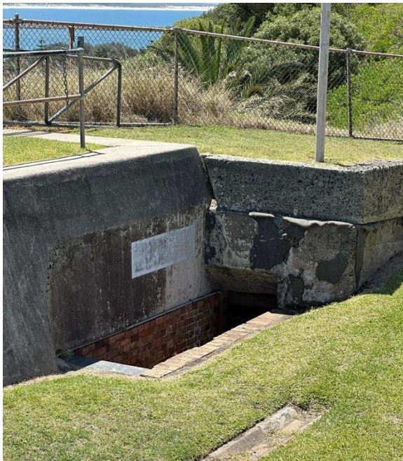
Figure 79. View to Mine Firing Station entrance from the dry ditch. (Source: CPH, 2024)
