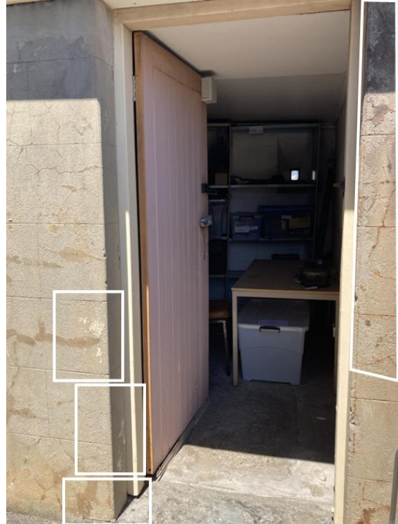
Figure 204. Delaminated render and efflorescence are present on the NCOs' Ablutions block exterior. (Source: CPH, 2023)
