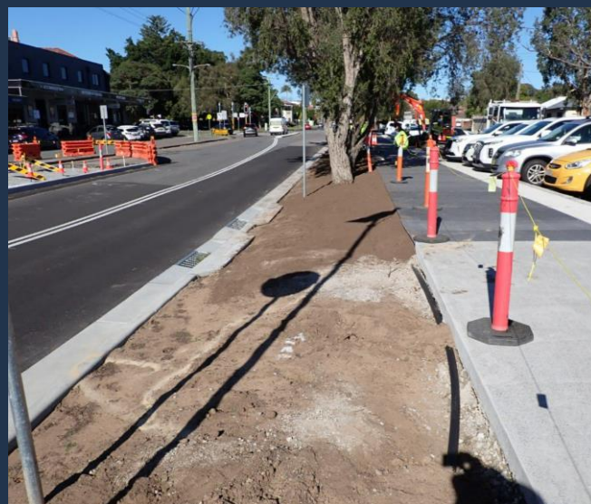
Underway: Road and drainage upgrades at Orchardtown Road New Lambton local centre.
