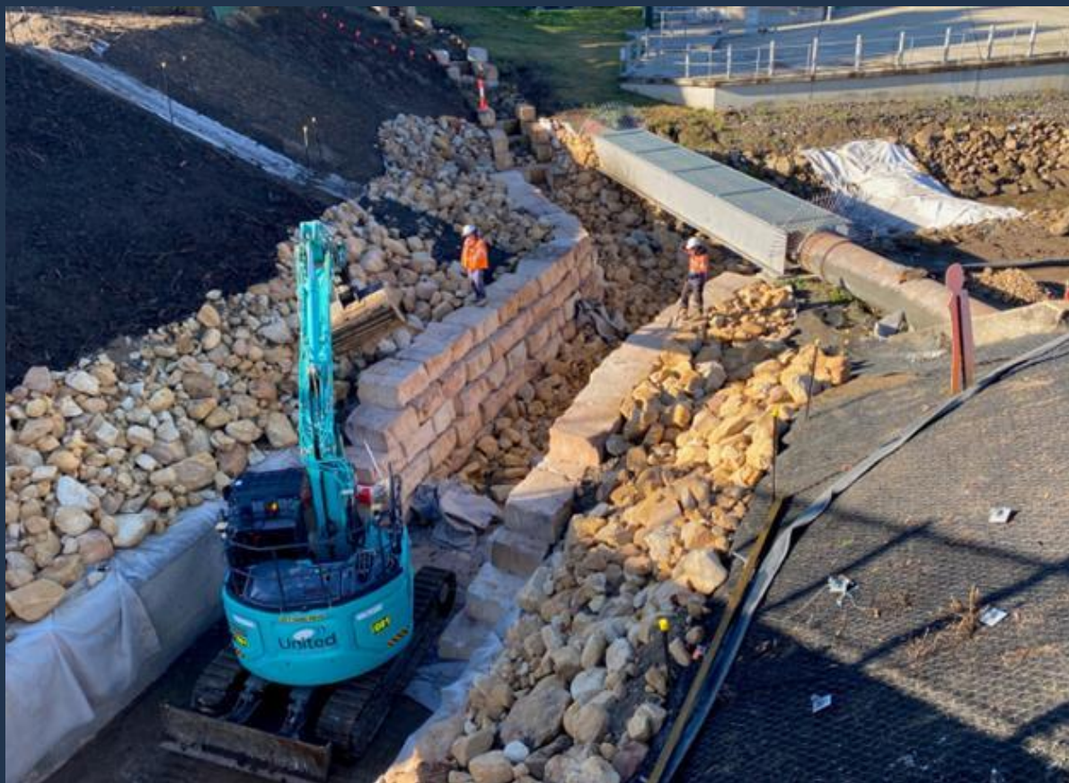
Underway: Stormwater improvements and new footbridge at University Drive Waratah West University Drive Catchment Rehabilitation
