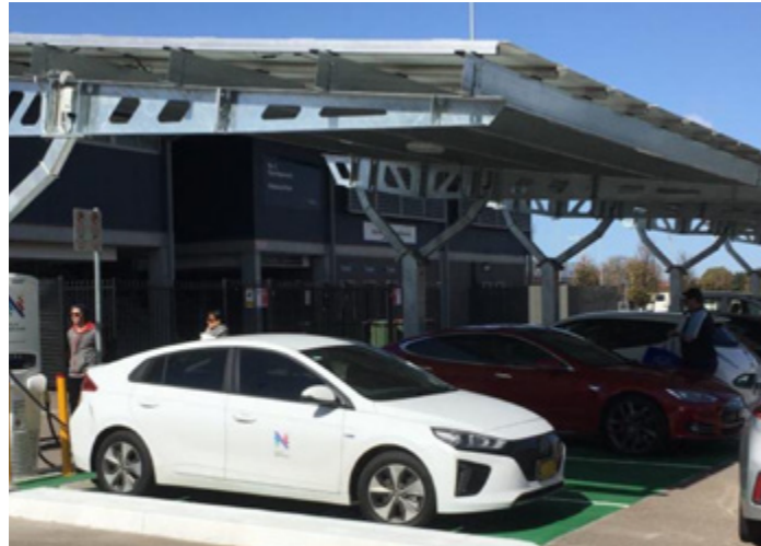
Solar panels above EV charging station at No. 2 Sportsground
